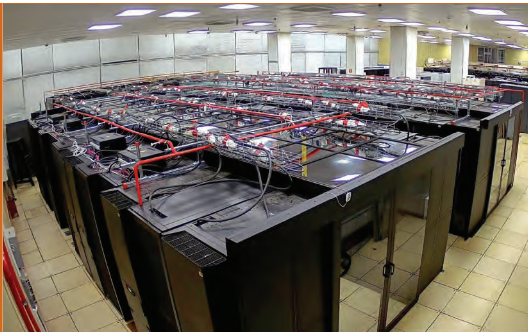
Top view of upgraded Modules 1 and 2, transferred to the cold corridor cooling with inter-row air conditioners, in the MICC machine hall
