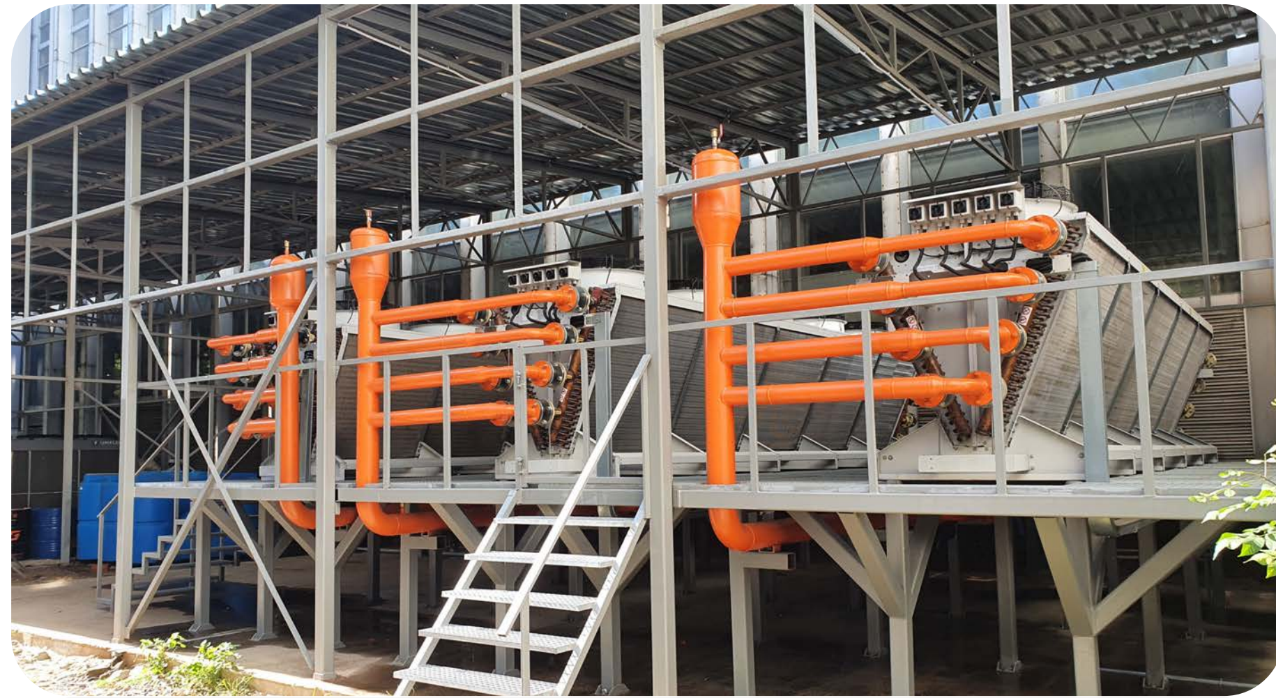
Dry cooling towers of the MICC cooling system
