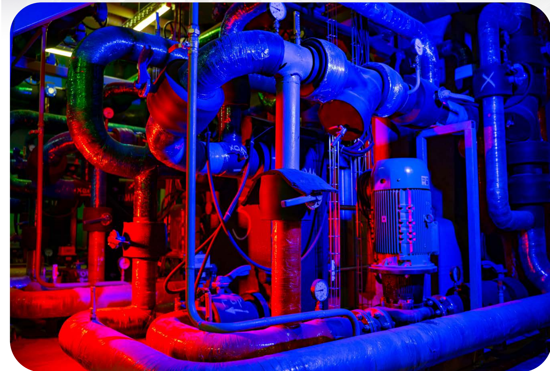
Dry Cooling Tower Pump and Heat Exchanger
