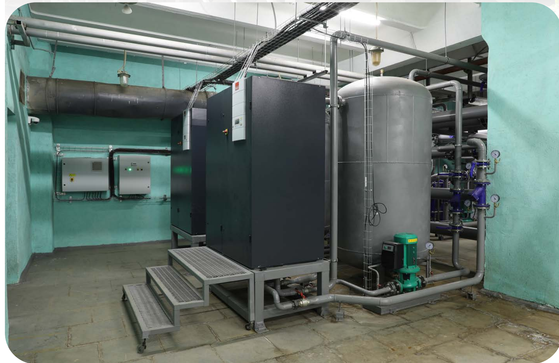
Refrigeration machines of the MICC hall
