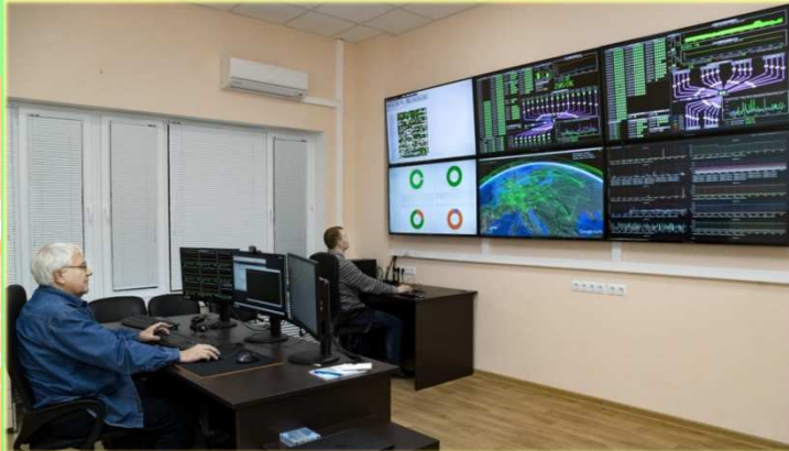
Figure 1. Photo of the MICC Operation Center
